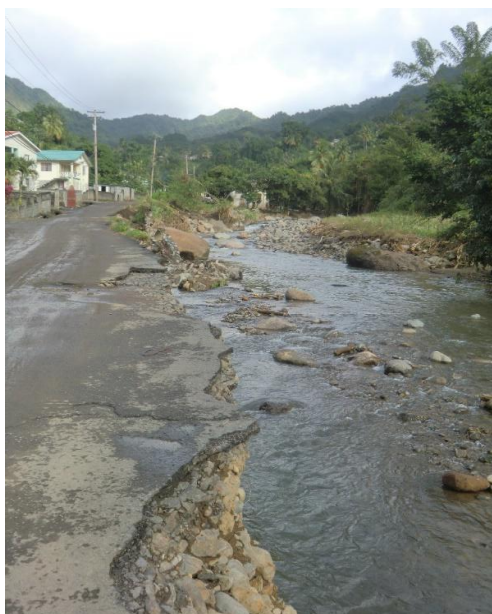
Figure 83. The Buccament River, Vermont, on 11 th January 2014, showing erosion of the bank and scouring of the riverbed caused by the 2013 Christmas Eve Flood.
